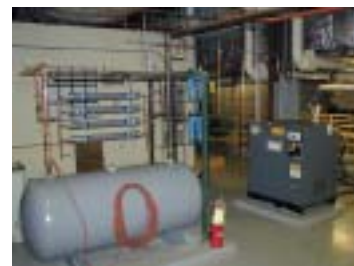
Membrane Air Dryer. Photo by Ron Crawford.
