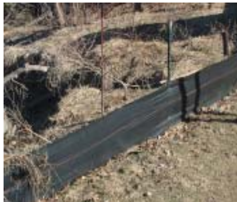
Silt Fence: Use silt fences, plastic sheeting and drain covers at construction sites
